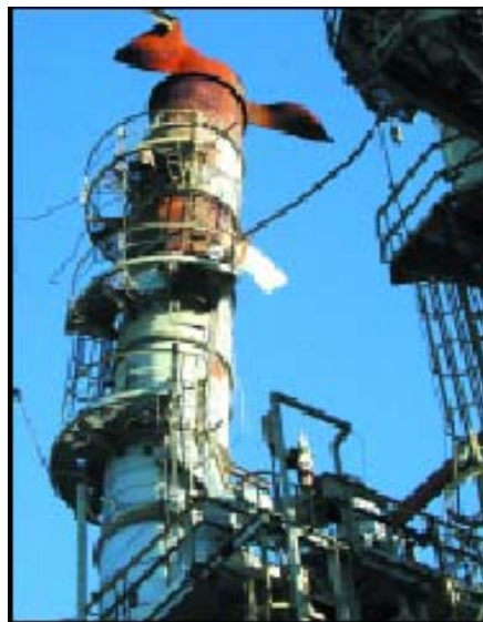
This accident investigated by and picture provided by the U.S. Chemical Safety and Hazard Investigation Board. Visit their site at http://www.csb.gov
