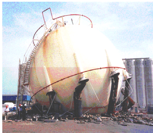
Corrosion Attacks Structural Supports
