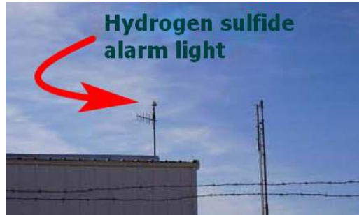
Fig. 2: H 2 S alarm warning light
