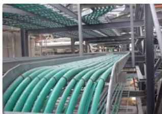
Cable trays and carriers
