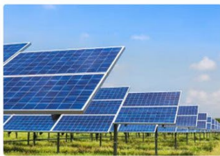
Solar Panels and Solar Farms
